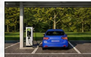
EV CHARGING STATION
